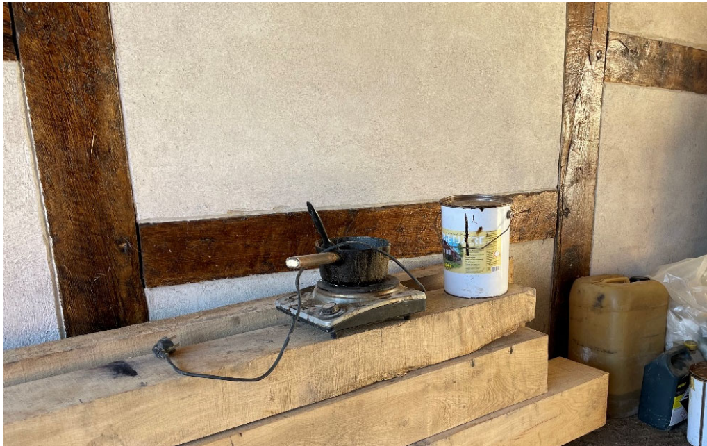
Heating the wood tar in a pot on an electric hob. Look at the brown color of the freshly spread, hot wood tar on the half-timbering behind.
